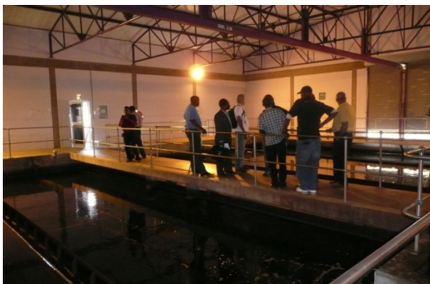
Field Trip: Goreangab Water Reclamation Plant
