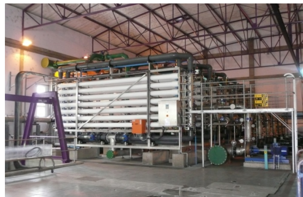
Field Trip: Goreangab Water Reclamation Plant
